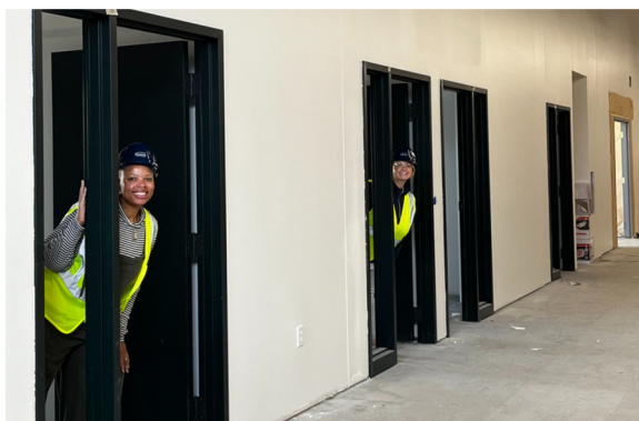
Paint and lights are really transforming things at the new Community Food Center!
